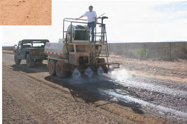
Photo 14. Applying synthetic fluid to road surface using distribution bar on rear of HydroSeeder
